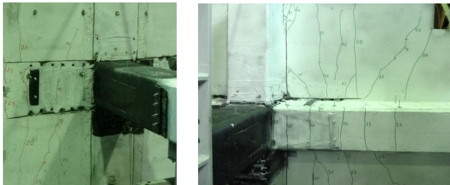
Fig. 7. Final damage state in C1-RT-B; left: column and slab, right: beam underside
