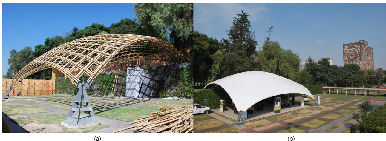
Figure 6. Bamboo pavilion during construction (a) and in service (b) at the National University of Mexico in 2010
