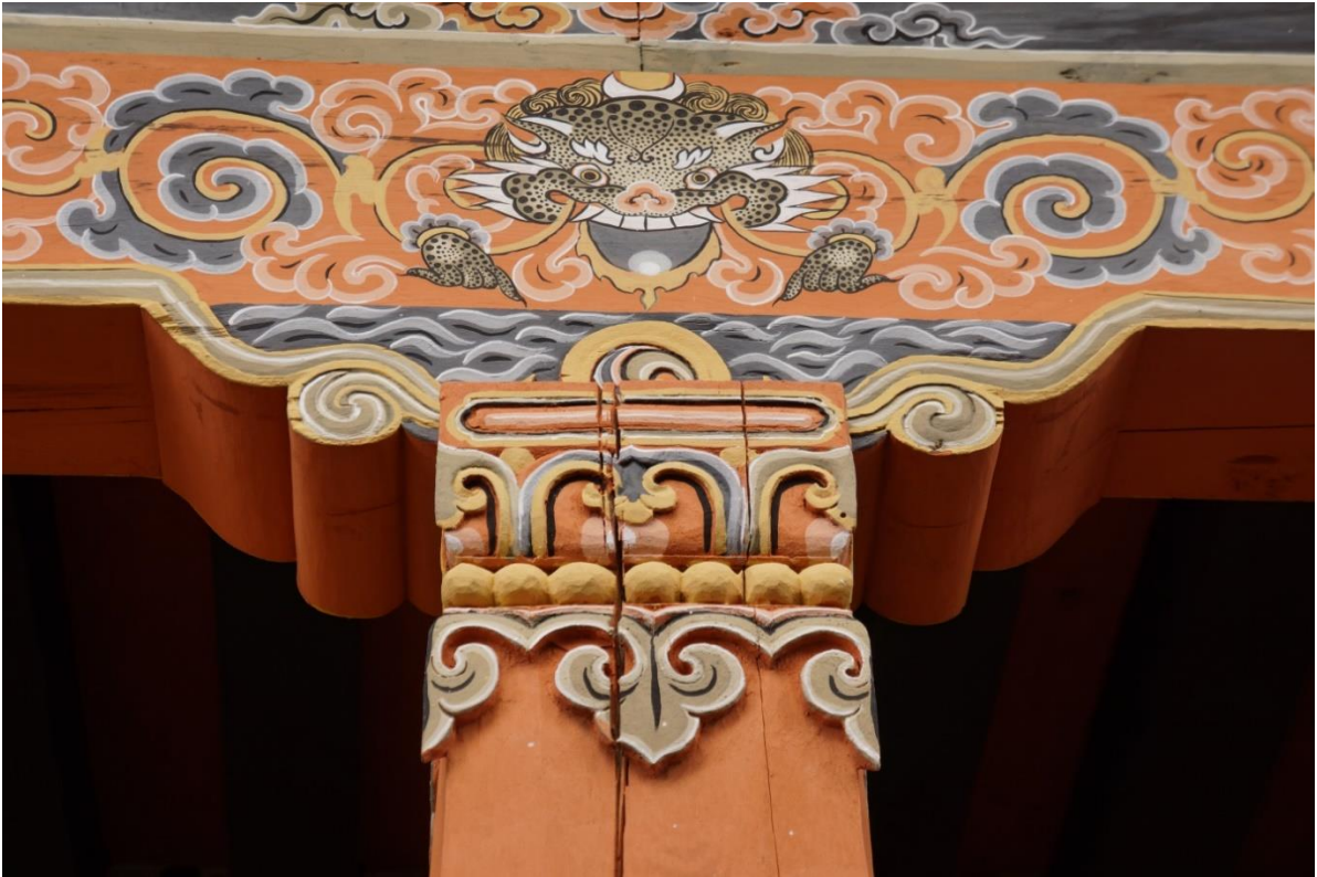
Figure 21. Simtokha Dzong: the replacement of timbers, with some issues of timber preparation, and highlighting the need to maintain wood carving and painting skills.
