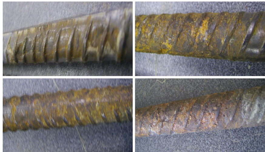
(b) Corrosion of the anodic steel bar (top left is PC concrete and the other ones are AAS concretes)
