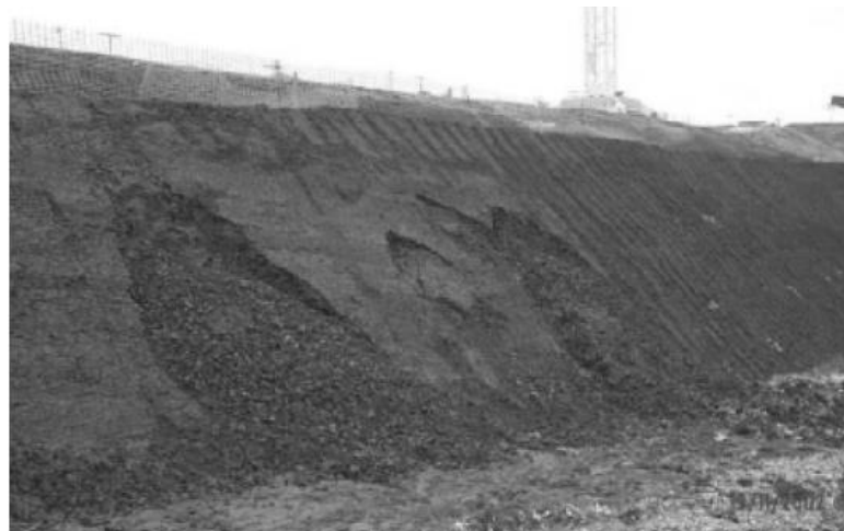
Figure 2-47. Shallow slope failures in Heathrow Terminal 5.(Hight et al. 2007)
