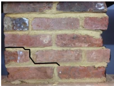
Figure 3: Failed masonry wallette showing location and extent of shear crack
