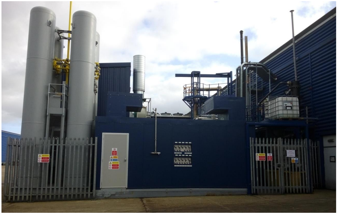
Figure 2.7.3. Pilot Plant of the Gasplasma process developed in Swindon for Bio-SNG production.
