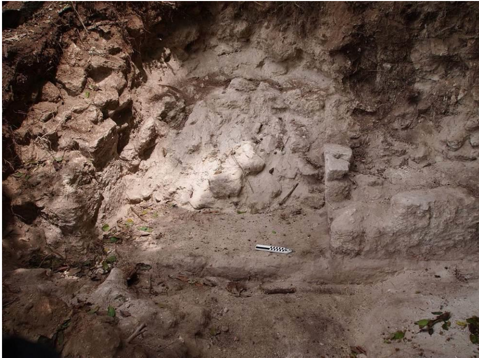
Figure 190 Photograph of Str. TM-2 Collapse in doorway
