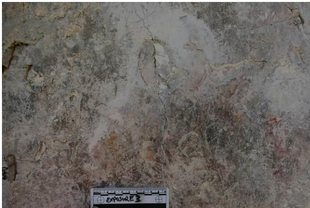
Figure C3: Photograph of painted area 3 West Wall, Str. TM-2
