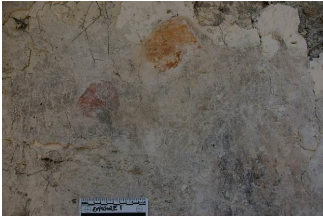
Figure C1: Photograph of painted area 1, West Wall, Str. TM-2
