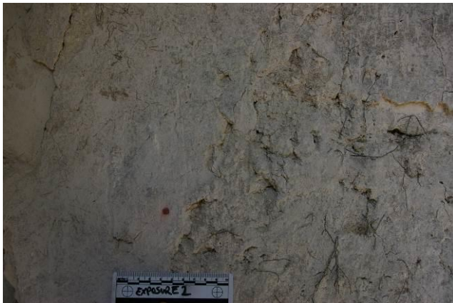
Figure C2: Photograph of painted area 2, West Wall, Str. TM-2
