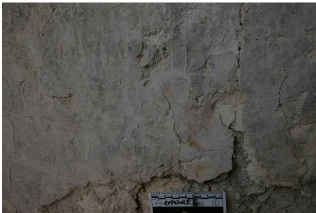
Figure C6: Photograph of painted area 6 West Wall, Str. TM-2
