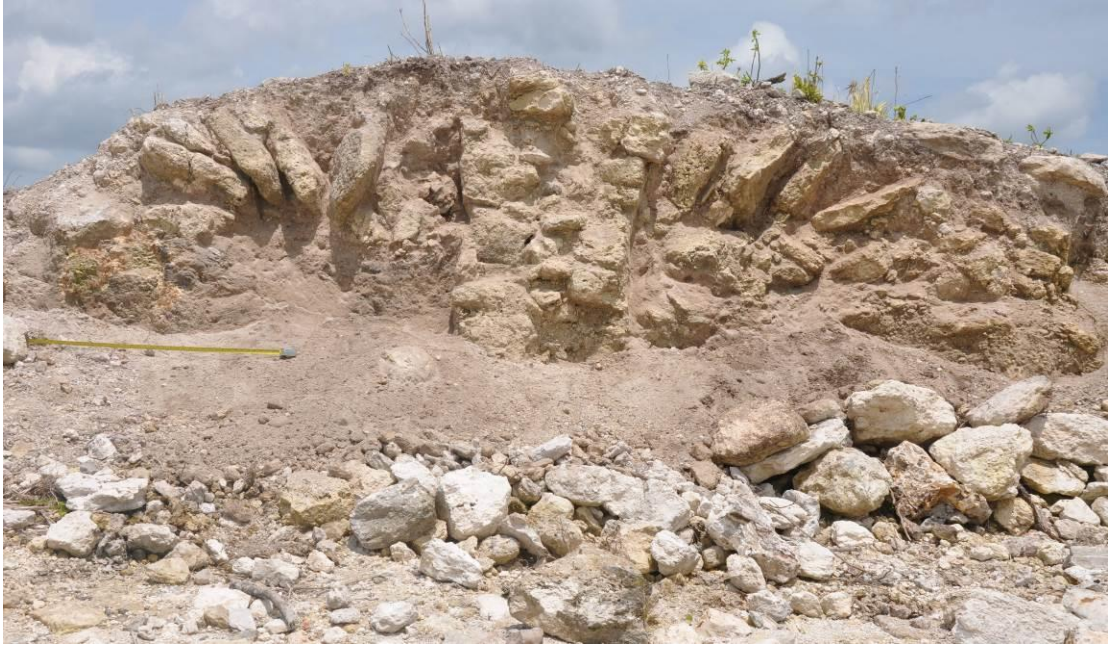
Figure 86 Photograph of collapsed vaulted roof, NOS11-M1
