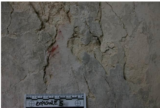
Figure C5: Photograph of painted area 5 West Wall, Str. TM-2
