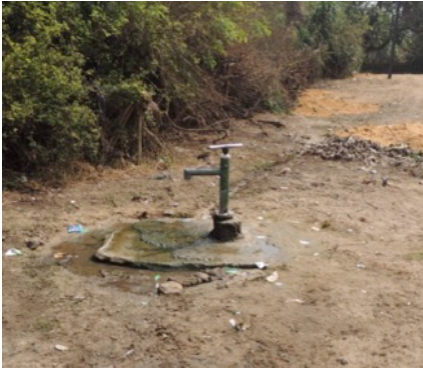
Image 6. 4: Deteriorating conditions of the water pumps in the island village (Image: Khirisahi, 27-10-13)
