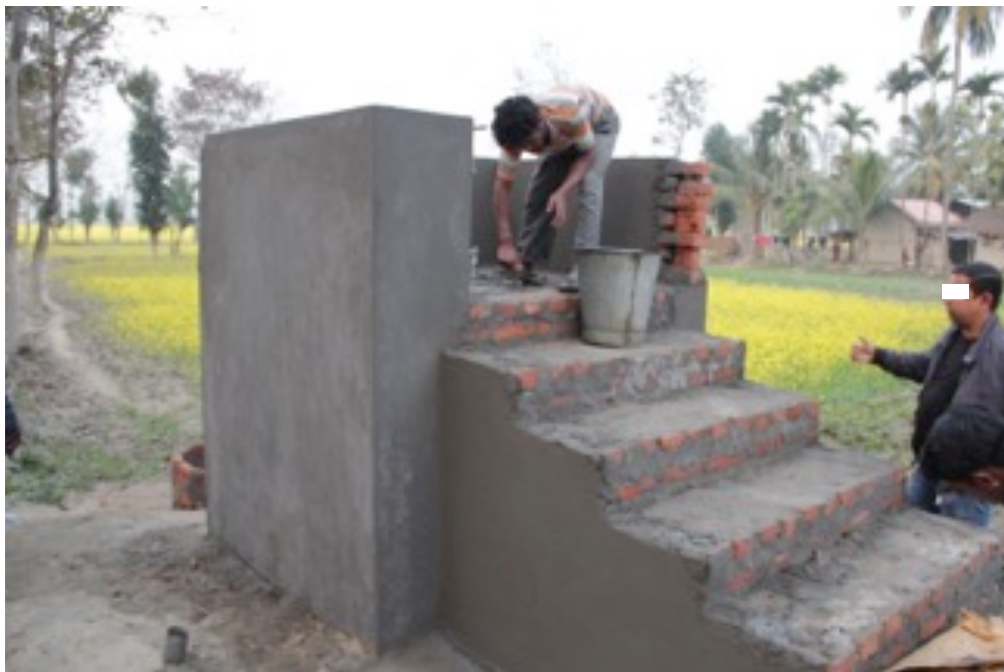
Image 5. 23: Raised hand pump by Agency AA (Image: Sonitpur, 17-01-13)
