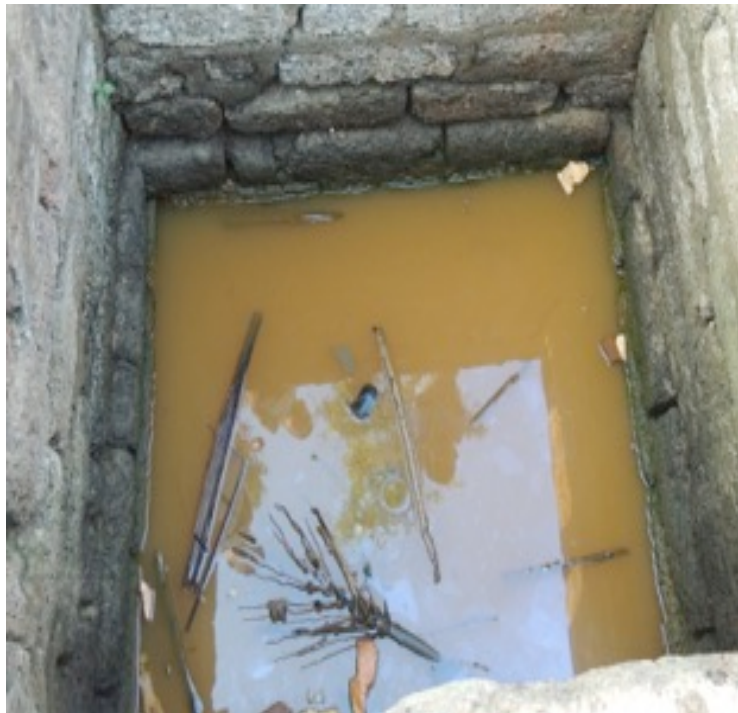
Image 6. 9: Open well with debris (Image: Sanpatna, 20-10-13)
