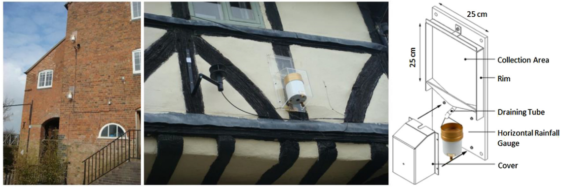
Fig. 3. WDR gauge designed and manufactured as part of project PARNASSUS on the facades of Abbey Mill and 1-Mill Bank, respectively.
