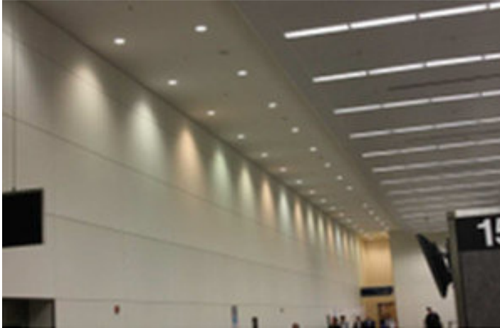
Picture 7.5: Lighting installation with low quality LED products that emit different colour of white light 26 .
