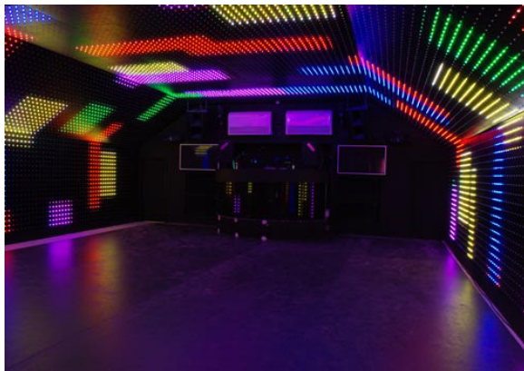
Picture 2.11: LED installation in Fire nightclub
