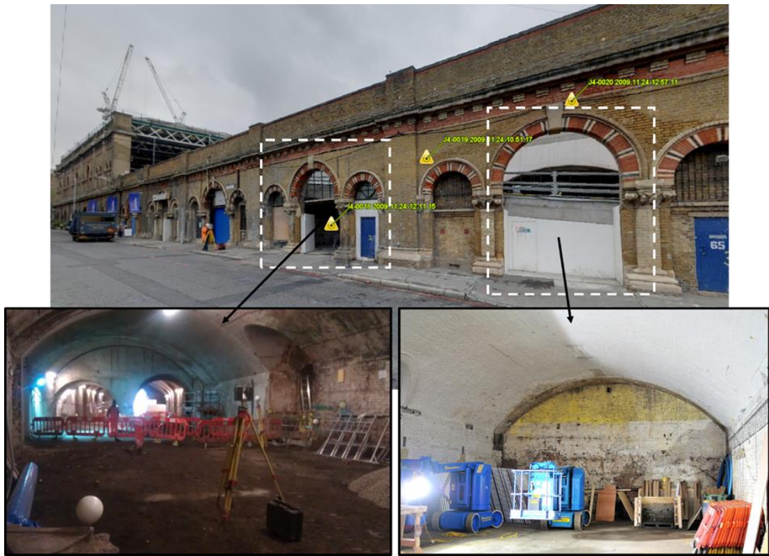
Figure 2.12: Examples of London Bridge Station arches (top image taken from NR TLP published TruView)
