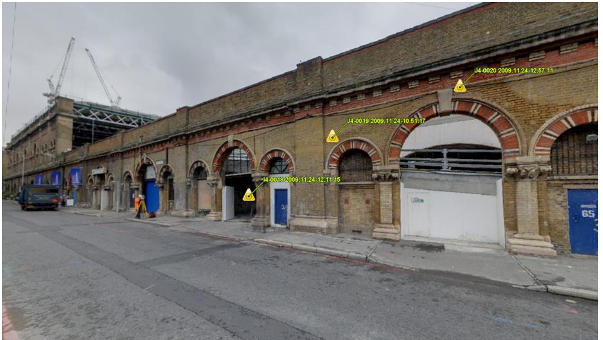
Figure 6.1 Image of London Bridge arches at street level with train shed visibly located overhead (image taken from NR TLP published TruView)
