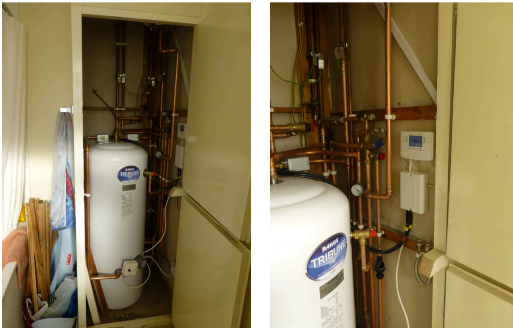
Figure 5.4 Hiding controls to satisfy electrical regulations.
