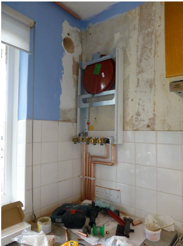
Figure 7.3 The uncomfortable frame for the new boiler, sitting in the shadow of the forsaken kitchen cupboard.
