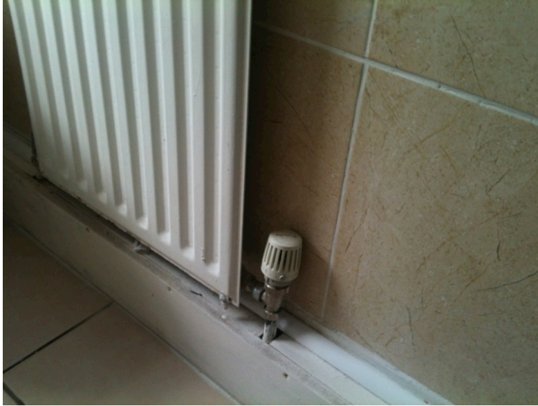
Figure 7.5 Radiators 'locked in' by boxes.
