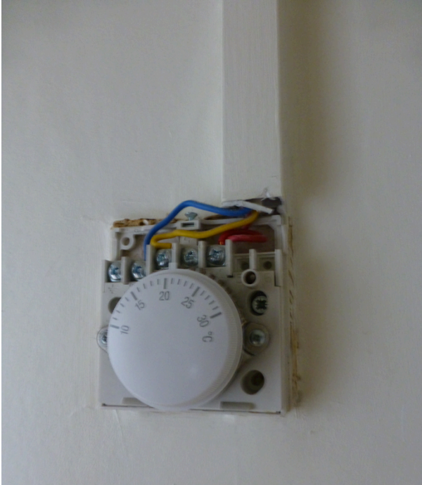
Figure 7.6 A well established room thermostat.
