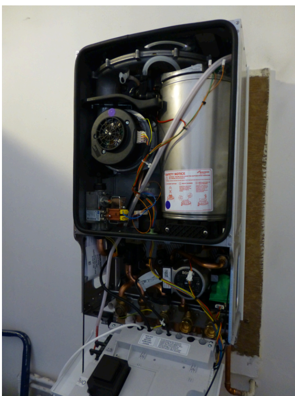
Figure 7.1 The exposed innards of a boiler.
