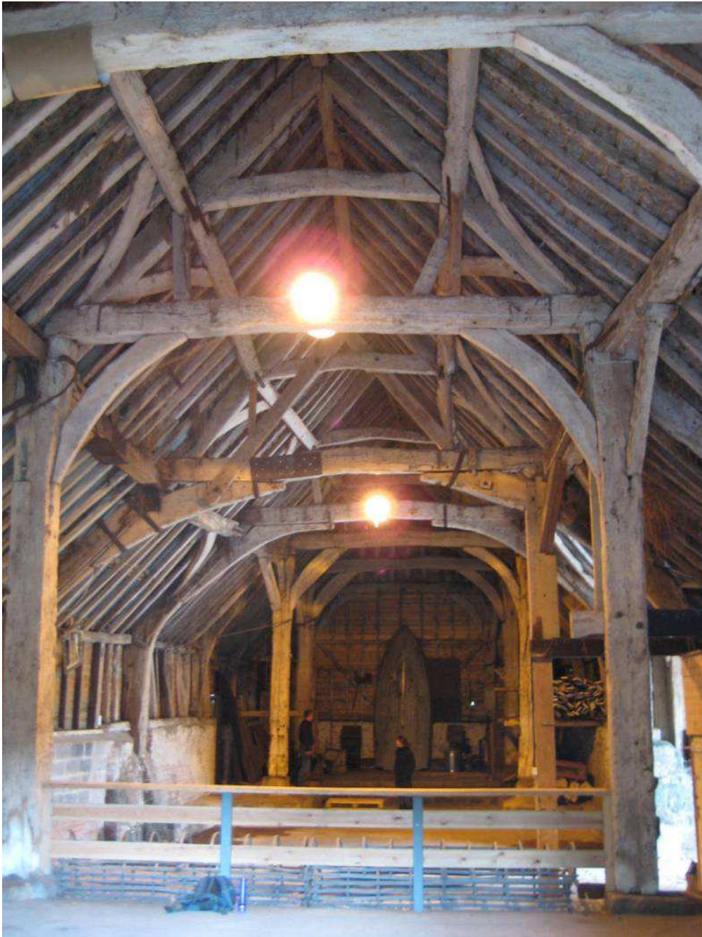
Figure 5: General view through the barn stood at Truss 2 viewed looking north (photo Matt Hurford)
