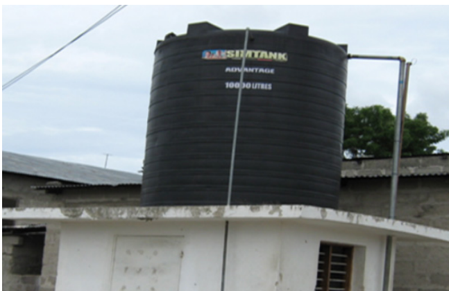
Image 4: Water tank installed by Plan International Source: URP, 2013
