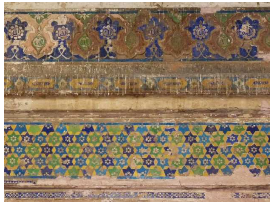
Figure 7.15 Tile-work decorating the interiors, as on the mihrab frame in the detail seen here, is in a much better state than that on the exteriors, very little separation of the glaze from the body noticeable.
