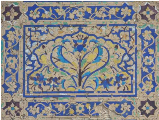
Figure 7.27 An intricate tile-mosaic panel on a wall surface. Highly ornate floral depictions, such as this one, dominate the tile-work compositions employed on this building.
