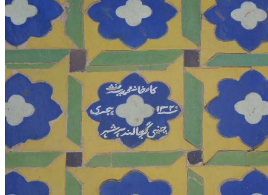
Figure 7.42 An inscription recording a past restoration event. Tiles in the vicinity of the inscription can be seen to be relatively inferior in make and in their laying technique.
