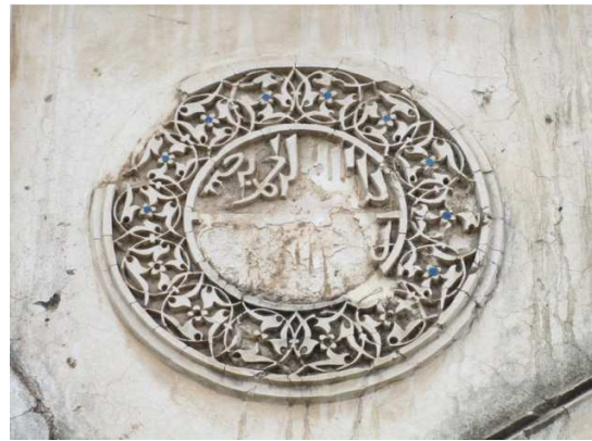
Figure 6.12 A stucco medallion on the spandrel of an arch on the mosque-structure, exhibiting tiny turquoise coloured tiles inset in the carving.
