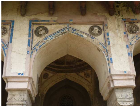
Figure 7.11 Detail of the tile-work on one of the verandah arches. The use of white coloured tiles can be evidenced here, employed in a mosaic composition with the two blues.
