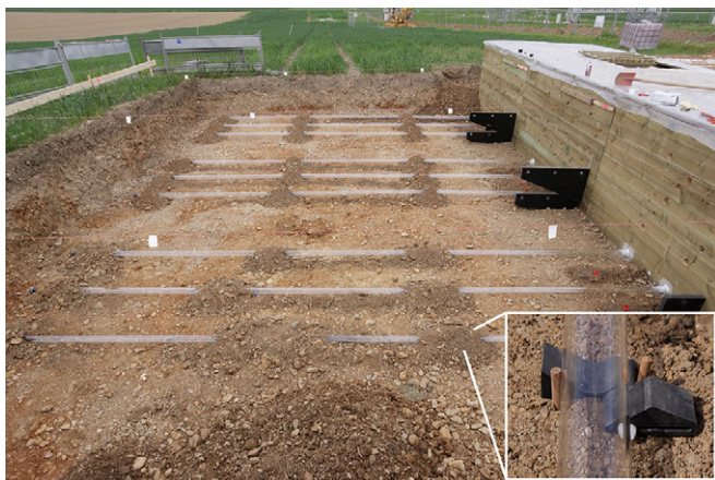
Fig. 1. Installation of the minirhizotron facility in the upper part of the test site. The wood container is the accessible facility. Wedge-shaped fixture blocks shown in the right corner were used to fix the tubes during soil backfill.
