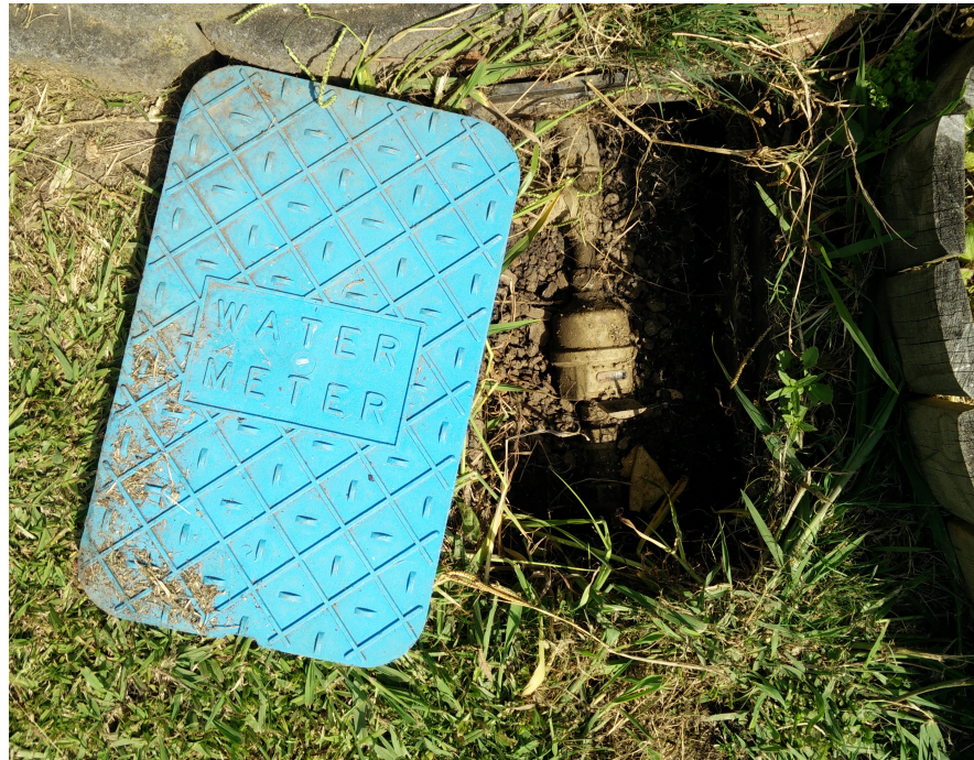
Figure 4.1: Photo showing a domestic water meter, and installation, (Kent PSMT 25mm) typical of an Auckland residential area.
