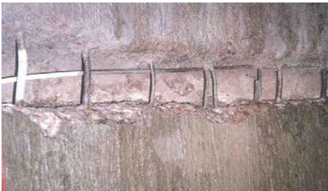
Figure B 3 One of damage conditions of shaft lining (from Liu et al., 2007).
