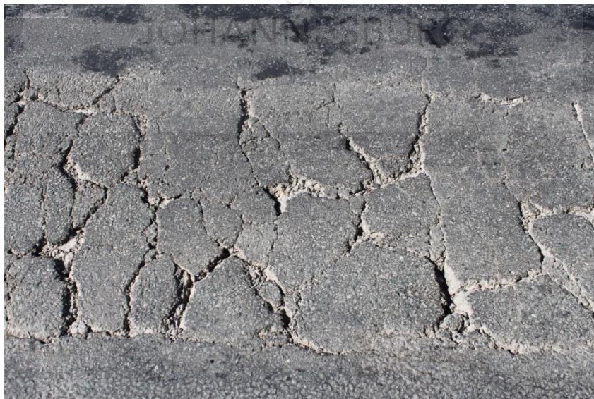
Figure 4.15: Fatigue cracking along the R59.
