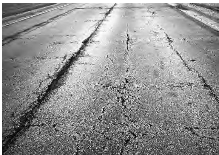
Figure 2.5: Longitudinal cracking on the road surface (source: Walker, 2002:9).
