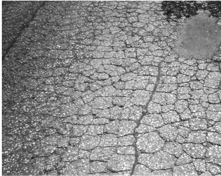
Figure 2.4. Fatigue cracking on the road surface (source: Walker, 2002:11).
