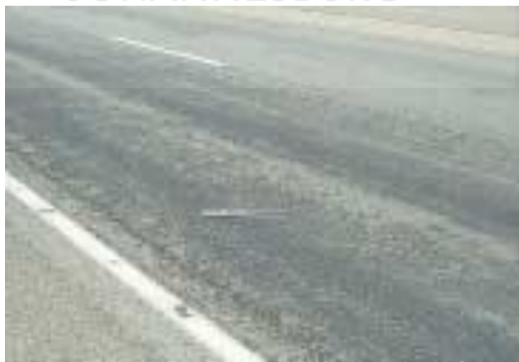
Figure 2.18: Bleeding of a road surface (source: US Department of Transport, 2003:26)
