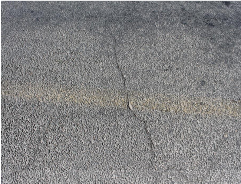
Figure 4.14: Transverse cracking of the pavement.
