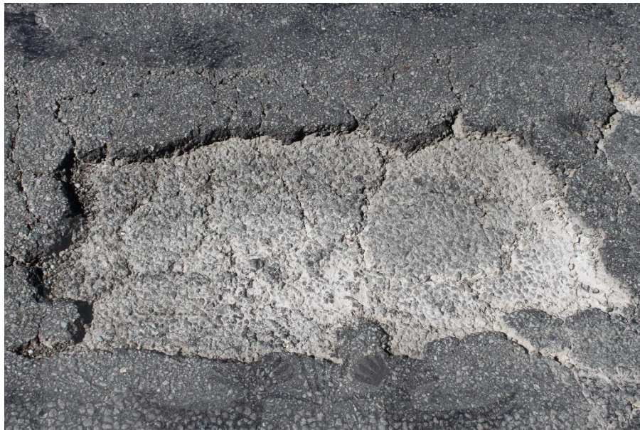
Figure 4.13: Photograph of pothole forming on the R59.
