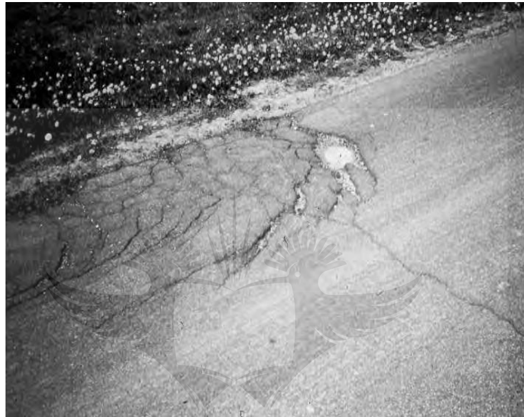
Figure 2.8.: Slippage cracking on the road surface (source: Walker, 2002:8).
