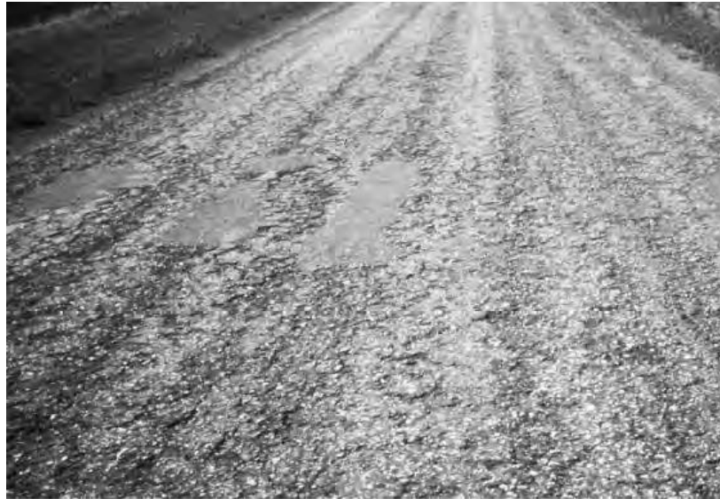
Figure 2.17: Ravelling of a road surface (source: Walker, 2002:4).
