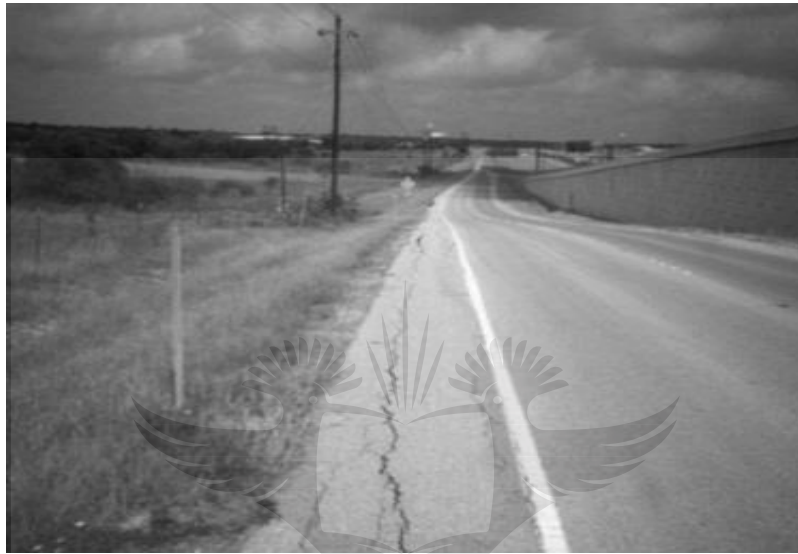
Figure 2.10.: Edge cracking on the road surface (source: Walker, 2002:11).
