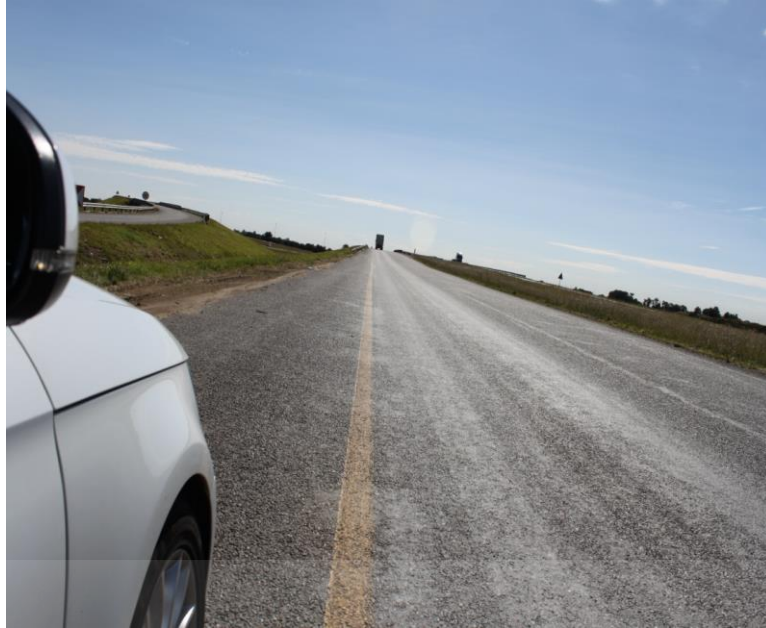
Figure 4.17: Bleeding along the surface of the R59
