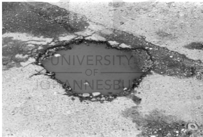
Figure: 2.15: Pothole in road (source: Walker, 2002:13).
