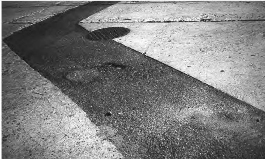
Figure: 2.16: Patches on road (source: Walker, 2002:12).
