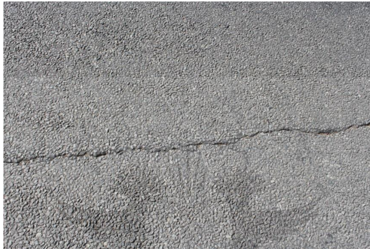
Figure 4.16: Longitudinal cracking found along the R59
