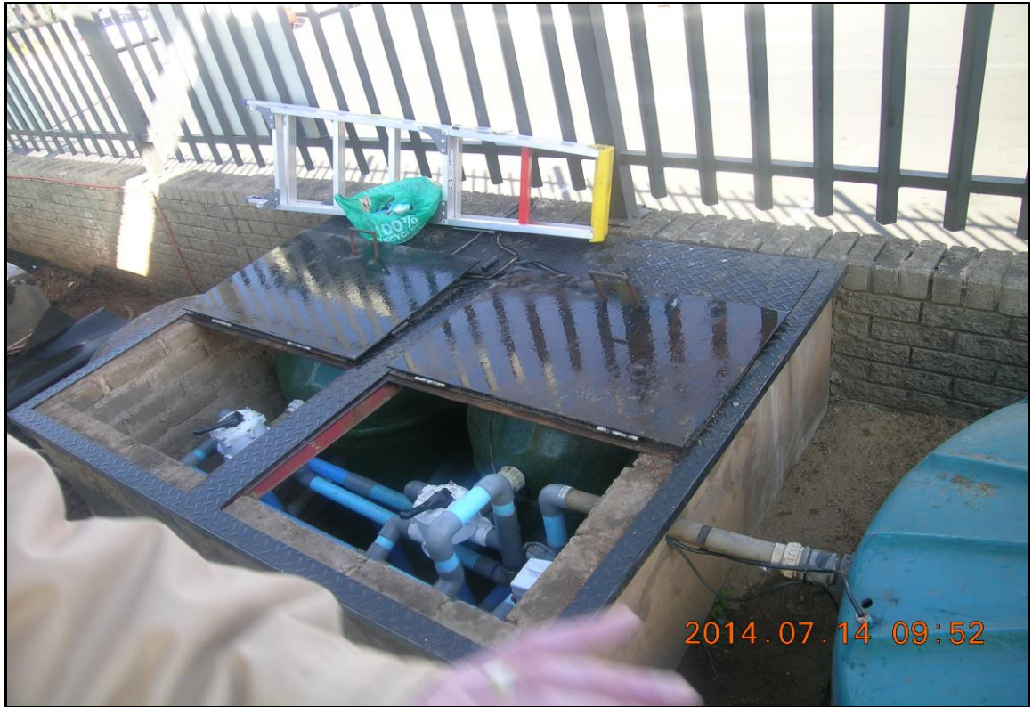
Figure 13: Wastewater recycling system in a carwash facility (By author)
