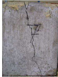
(b) Enclosing concrete splitting
