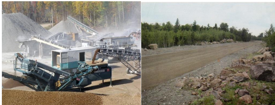
Figure 3: Quarry rock mined near the construction site is processed. Figure 4: Aggregate base course is constructed.
