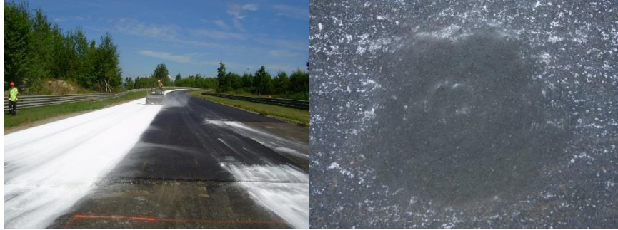
Figure 10: Hydrated lime is applied and rolled. Figure 11: tire mark generated by heavy loaded truck to check the stiffness of HMA surface after approximate one week of paving.
