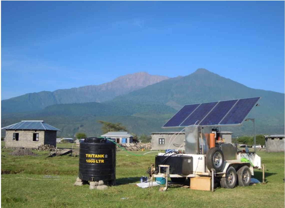
Figure 2.5: Photo of ROSI installed at Ngare Nanyuki, Tanzania
