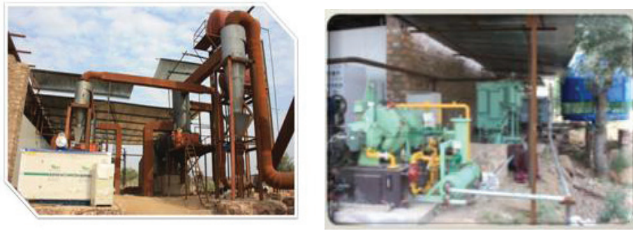
Fig. 4: Biomass Boiler, Turbine and VAM Set Up
