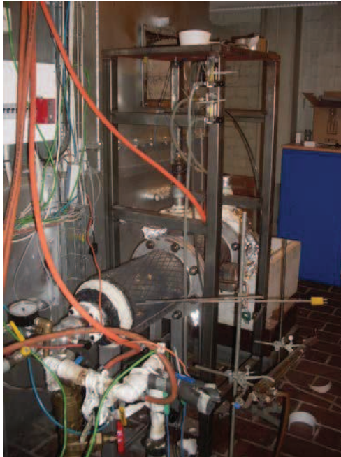
Figure 23. Gasification device without insulation.
