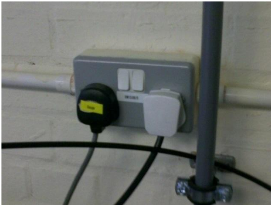
Fig.5 Power supply for barometer and pump
