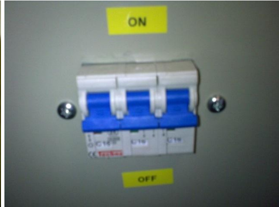
Fig.4 Switch for main power supply
