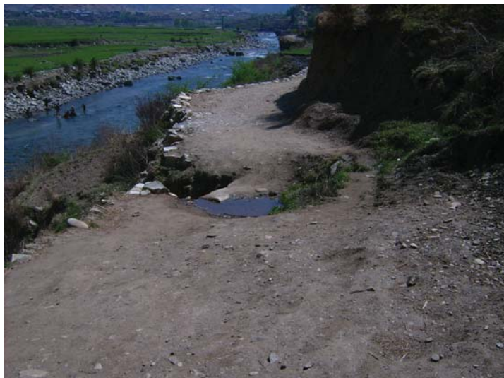
Picture 5: Road/track section damaged because of poor drainage structures, Kartikswami
