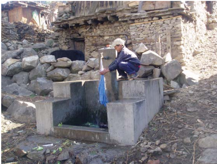
Picture 10: Well functioning tap, part of drinking water system, Dandafaya
