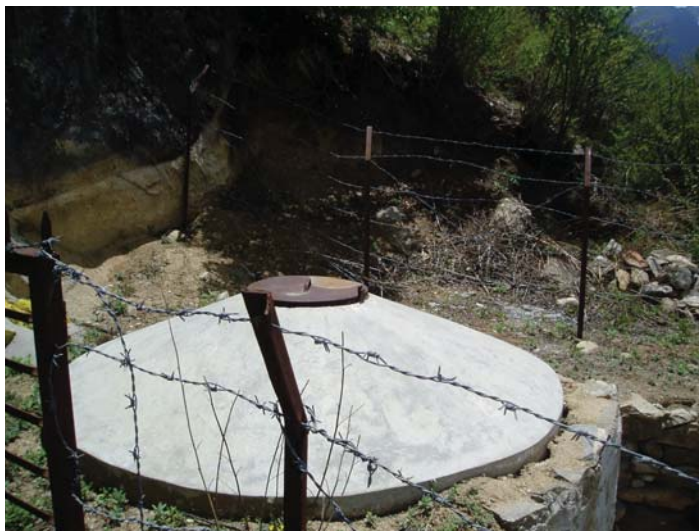
Picture 9: Reservoir tank for drinking water system, Dandafaya
