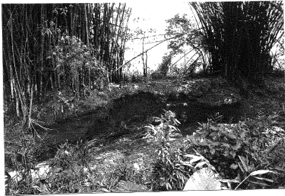
Figure 5.4 Undercutting of the Bamboo Planted to Control Bank Erosion of the Rio Cobre in Lluidas Vale.
