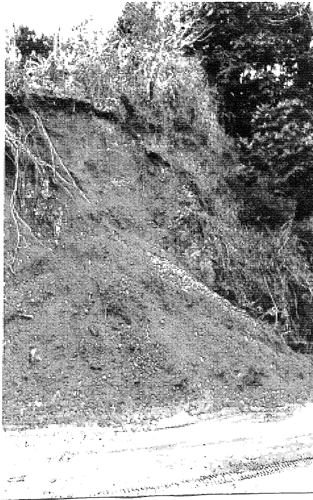
Figure 9.2 Slumping of Road Cutting Below Small-holder Cultivation
