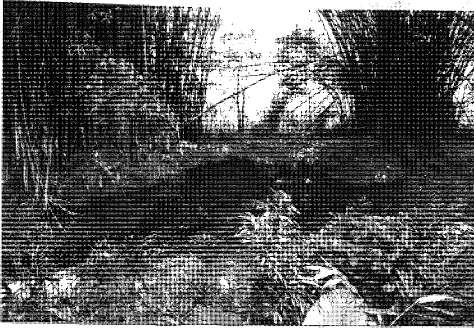
Figure 6.3 Undercutting of the Bank of the Rio Cobre in Lluidas Vale.
