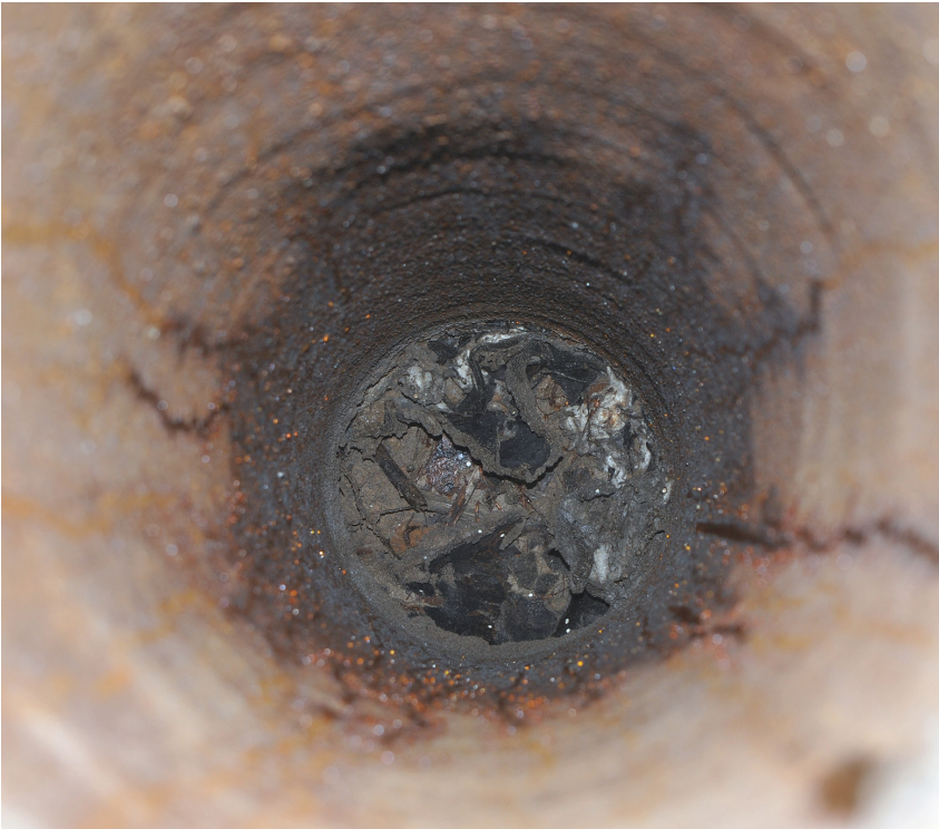
Figure 5. Bottom sight of the ventilation pipe outlet. Photo taken on 21.02.2016 (Wojciech Stephan).
