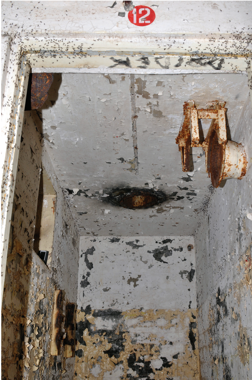
Figure 3. The upper part of the bunker space with the F. polyctena 'nest'. In the middle of the ceiling, the input of the ventilation pipe. Ants climbing walls (and hardly reaching the ceiling) en masse within and outside the room are visible (especially well on the door frame). Photo taken on 24.07.2015 (Wojciech Stephan).
