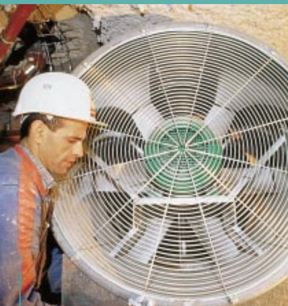
A recent example of Sophiane's know-how in air treatment: the smoke evacuation system for the new cardiology centre at the Pitié-Salpêtrière hospital in Paris.
