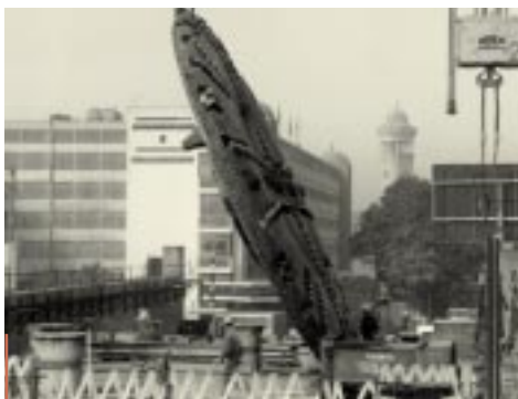
After leading the civil engineering works on line 2 of the Cairo metro, Campenon Bernard SGE is boring two road tunnels under the El Azhar district, the historic centre of the Egyptian capital.
