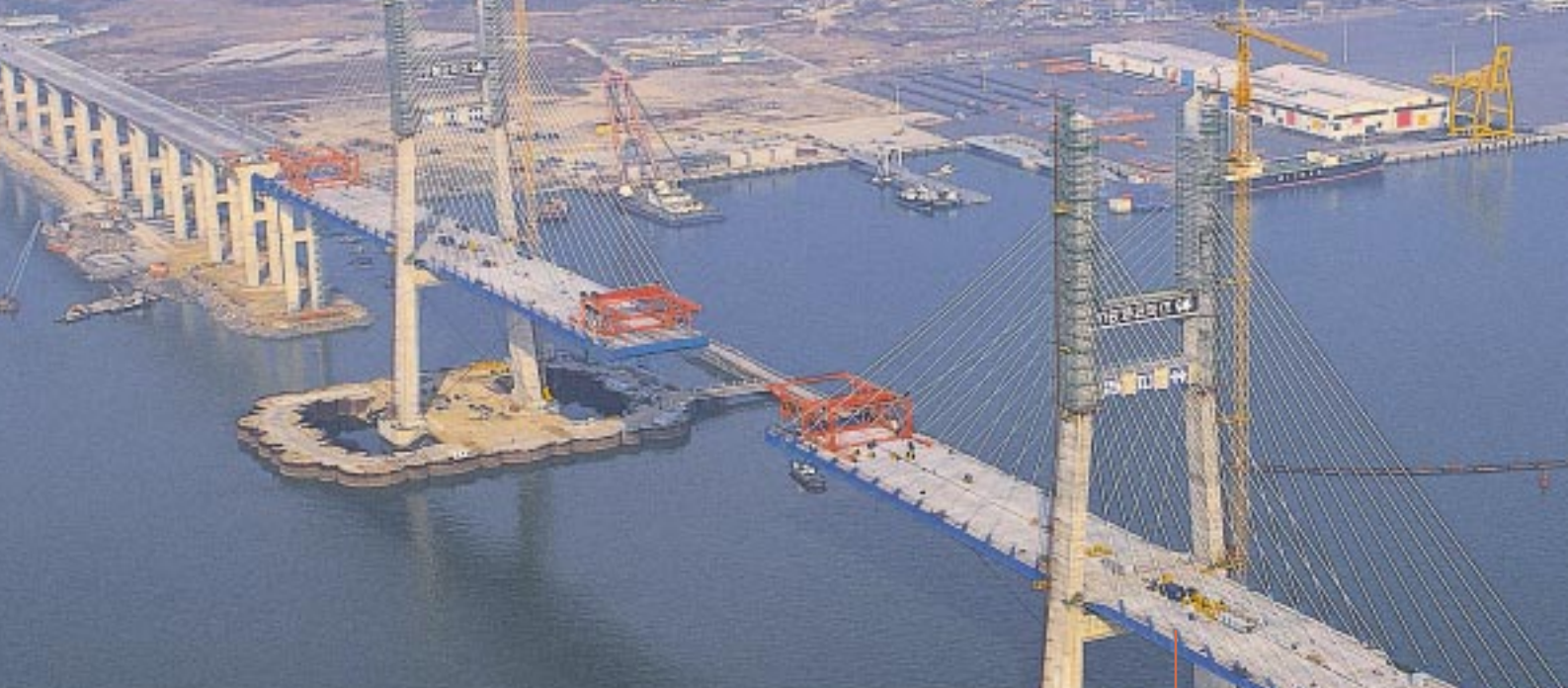
Freyssinet supplied the prestressing for pylons and stay cables on the Seohae bridge in Korea.
