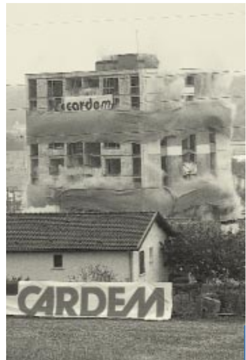
Recycling of demolition materials is today an ecological necessity. With Cardem, number one in France, and VBU, number one in Germany, Eurovia now has substantial expertise in this field.
