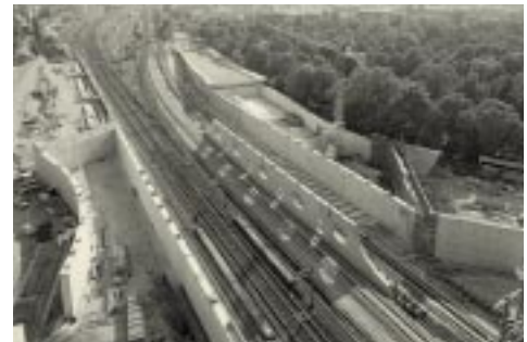
The «Berlin bridge» construction project over a railway line in constant use is the largest transport project in Leipzig since the Second World War.
