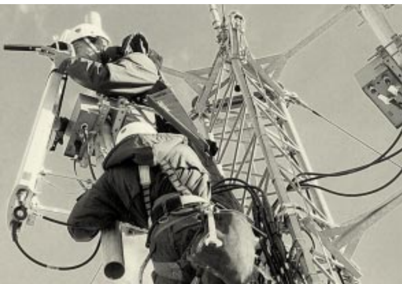
Through the Graniou brand, GTIE is working with the main mobile telephone operators as they deploy throughout Europe.
