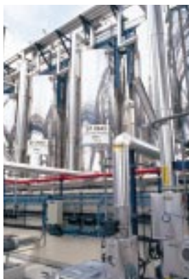
Villers-Saint-Paul facilities, Cray Valley
