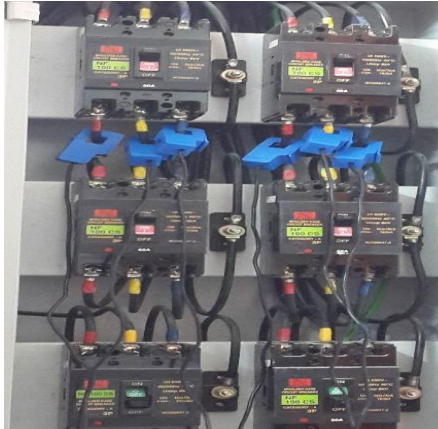
Figure 4: Six CTs connected at 3-phase air conditioner load
