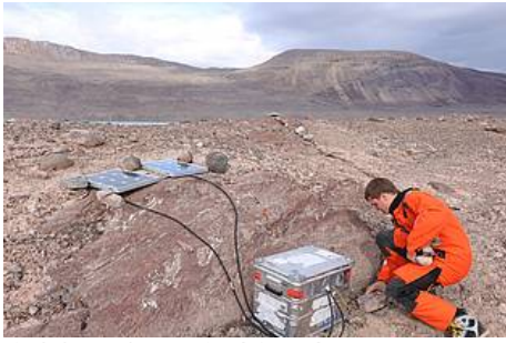
Fig. 2: Setup of the station CENT at Centrumssø. In the background the GNSS antenna can be seen while in the foreground the two solar panels and the Zarges Box with GNSS receiver, battery und a charging controller can be found. (Photo: Benjamin Ebermann)
