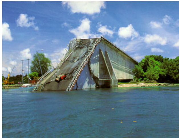
Figure 1.1. Collapse of K-B bridge after 18 years' service.
