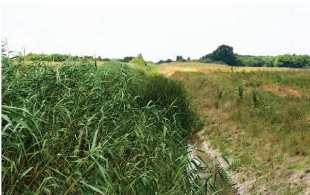
APPENDIX FIGURE 7. Small canal of second order (average width: 3 m) in Sombor municipality, Serbia.
