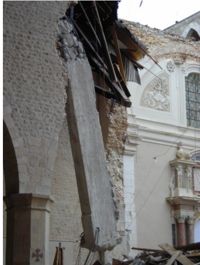
Figure 1.1 S. Maria di Collemaggio church: damage after 2009 earthquake showing the course of reinforced concrete inserted during the second half of '900
