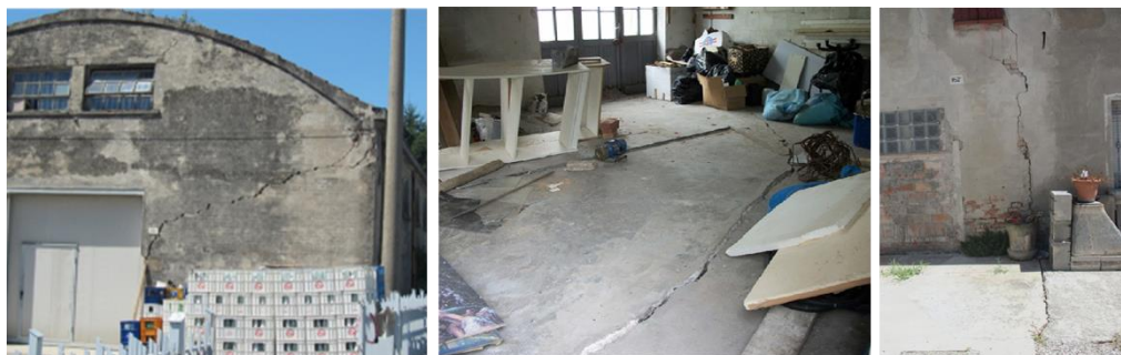
Figure VI.1.2 – Seismic-induced damages to structures on the crest embankment (Tonni et al., 2015)
