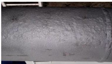
Figure 2 Example of external corrosion damage [12]
