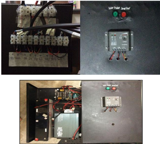
Figure 19 Controller Box Connection, Batteries, and Inverter
