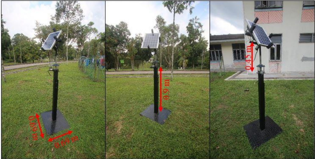
Figure 14 Different Angle View of the Solar Tracker Tower
