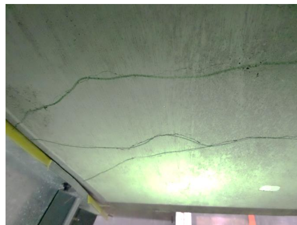
(b) Transverse cracks underneath slab M14 specimen
