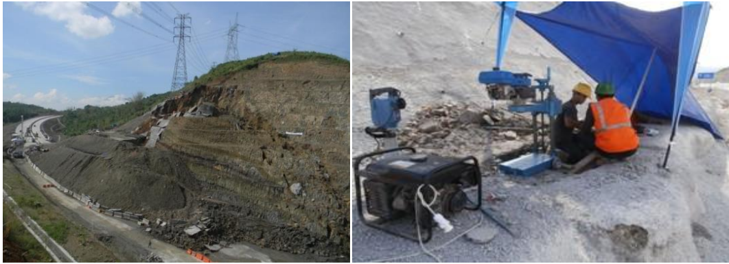
Figure 7 Landslide location at Semarang-Bawen toll road and test pit sampling work
