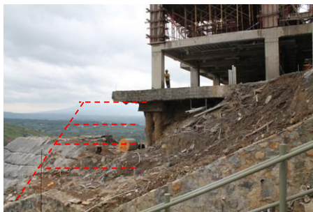
Figure 2 Landslide case in the Sport Training Center project at Hambalang Sentul, West Java [3]
