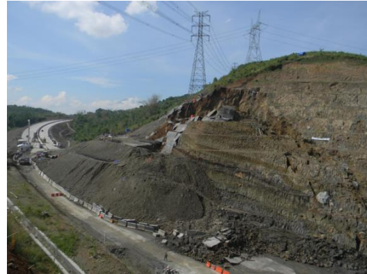
Figure 3 Landslide case in Semarang-Bawen Toll Road KM 32+000[4]
