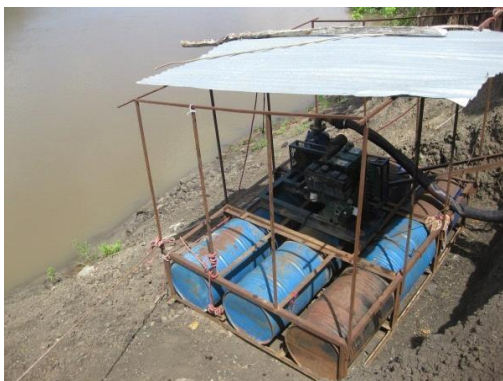
Figure 10. A good example of a solution to a problem – the floating pump station in Kakora. (Photo: Agnar Kjeller).
