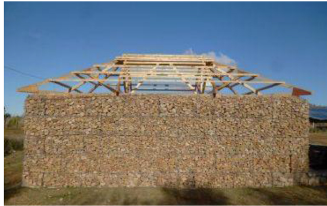
Fig. 3. 7 - gabion box house with timber roof, picture given by A&D (Architecture and Developpement)
