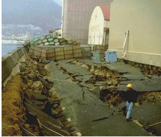
Figure 2.5. Liquefaction induced by earthquake (Kobe 1995)
