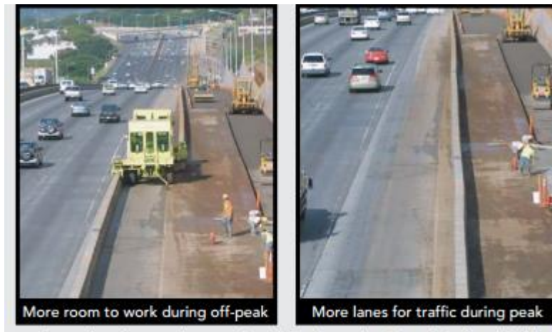
Figure 5-21: Use of moveable barrier system (Lindsay Corporation, 2015)
