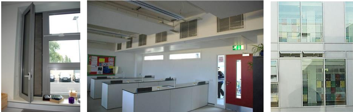
FIGURE 3. Building A cross ventilation strategy – top hung and secured side windows (left), plenum air intake (middle), and motorised vents on the corridor side (right)
