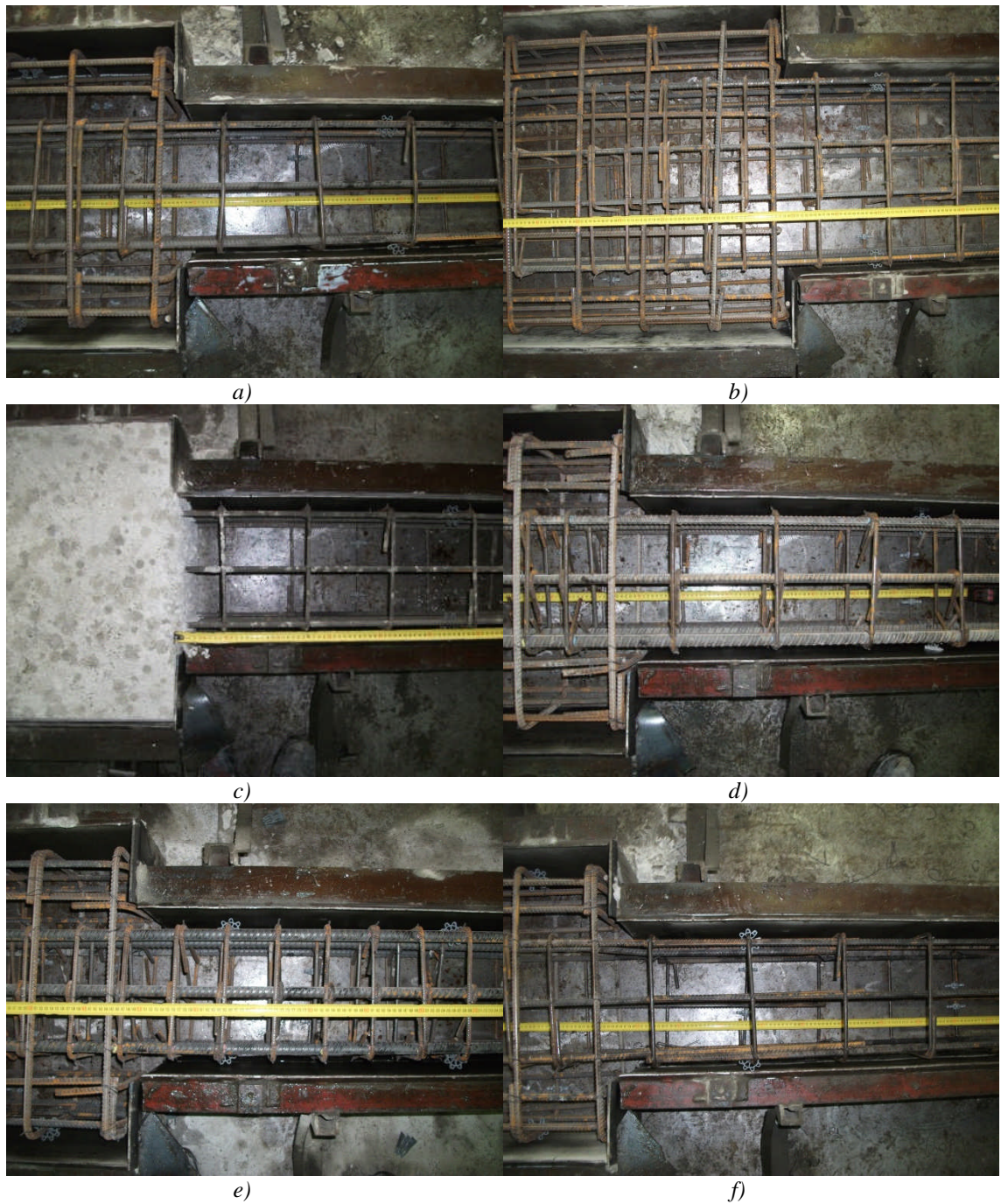
Figure 3-11 Details of the reinforcement layout and form work for various columns specimens: a) T14; b) T4; c) T6; d) T10; e) T12; f) T16-D1.
