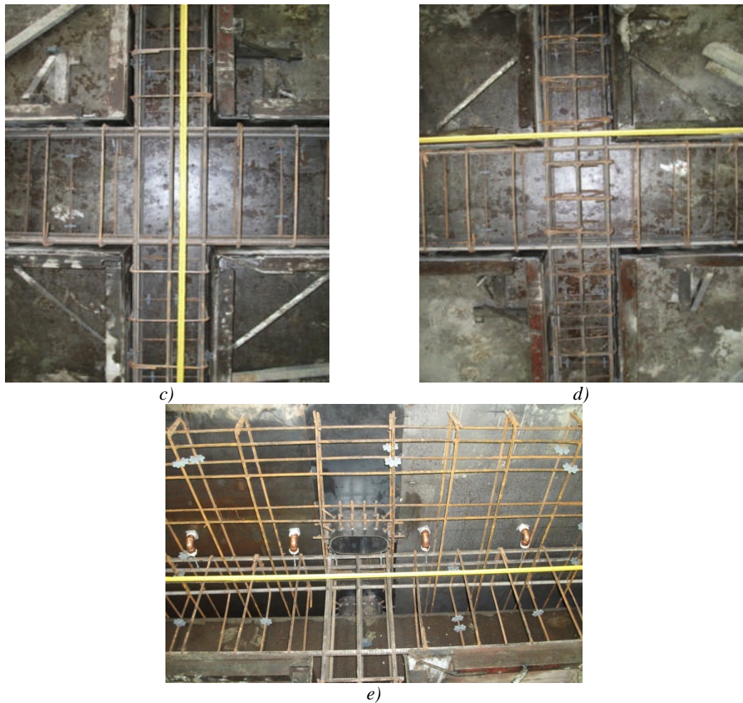
Figure C-4 Details of the reinforcement layout and form work for the internal beam-column specimens: a) J3-X; b) J5-X; c) J6-X; d) J7-X; e) J4-X
