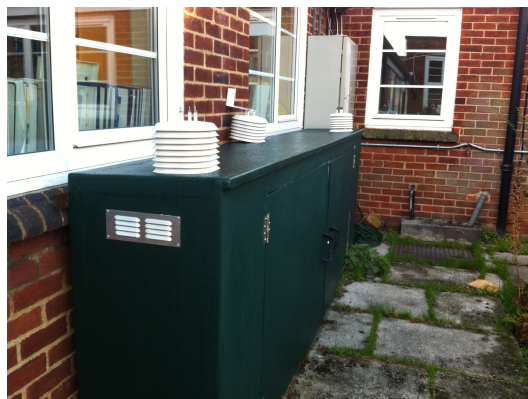
Figure 3.7: Stevenson screens installed in a school yard
