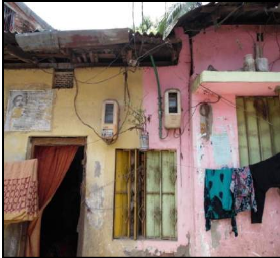
Figure 2.32: Electric meter is kept unprotected outside of the house, Chanmari bi lane, Motijhorna. Source: Field survey, August, 2014
