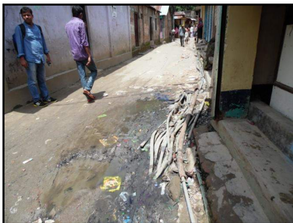
Figure 2.30: Poor management of water pipelines, Tankir pahar, Motijhorna area Source: Field survey, August, 2014
