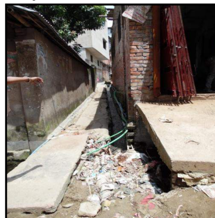
Figure 2.31: Co existence of drainage and water pipelines, Motijhorna hill, Motijhorna. Source: Field survey, August, 2014
